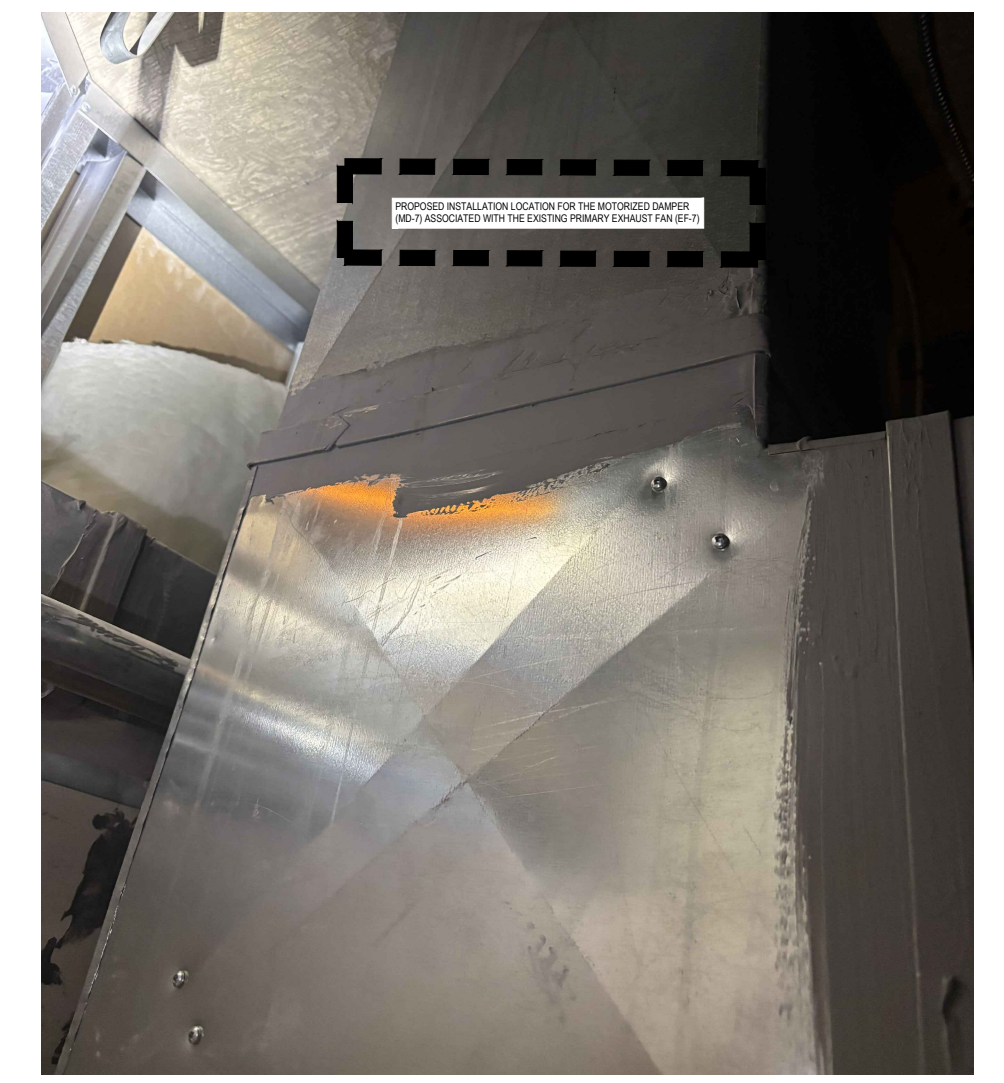
4 EXISTING EXHAUST AIR DUCTWORK IN PT W/C ROOM (1462) CEILING SPACE M-104 NTS
