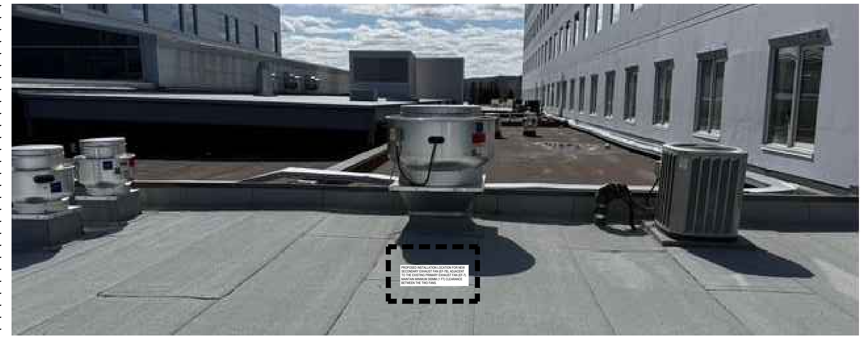
3 EXISTING MECHANICAL EQUIPMENT ON ROOF M-104 NTS
